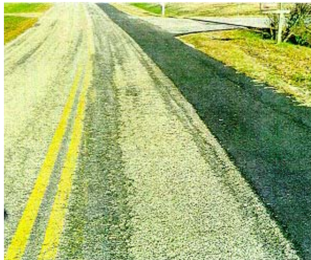
Figure 10. ACHM Pavement Showing Severe Ravelling.
